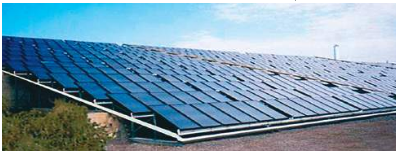
SARANTISS.A., 1999-Solar Air -Conditioning 700kw
